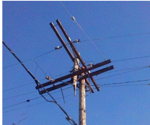
Figure 21: Typical LADWP Broken Wood Pole
