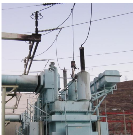
Figure 14: Example of an Old Substation Power Transformer
