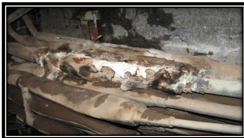
Figure 26: Example of Failed Underground Splice
