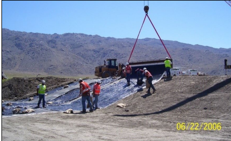
Figure 4. LADWP Construction Crews laying geotextile fabric at one of ten original measuring stations, June 2006
