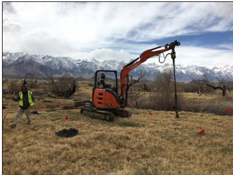
Figure 9. Drilling planting holes. Up to 30 poles, supports, and plant protectors were installed per hour
