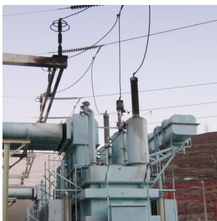
Figure 14: Example of an Old Substation Power Transformer
