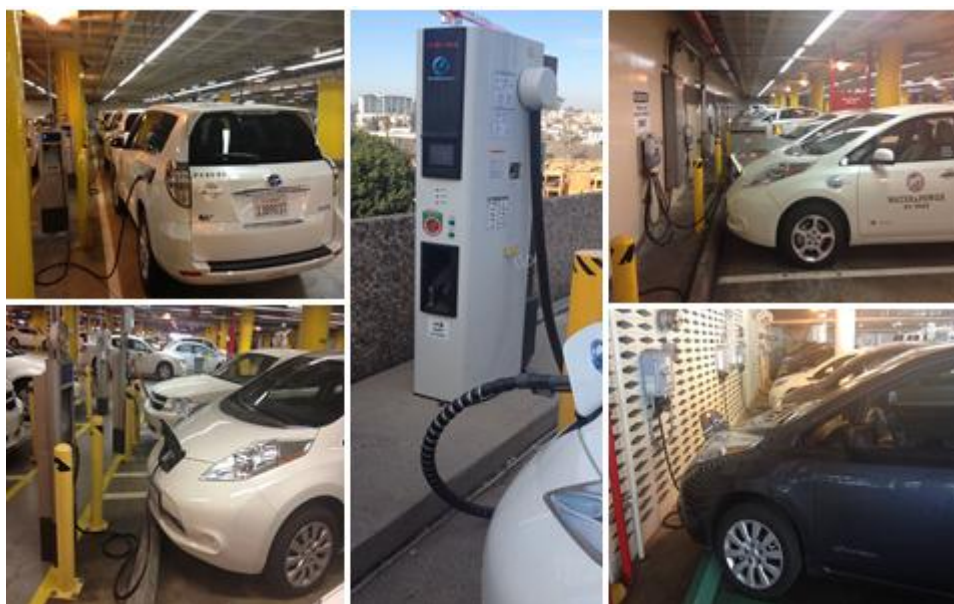
Figure 56: LADWP Fleet and Public Charging Stations Installed Across Los Angeles
