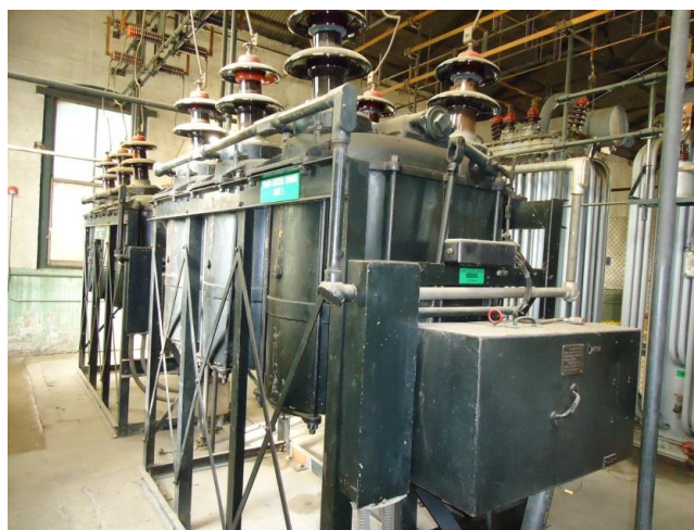
Figure 15: Example of an Old Oil Circuit Breaker
