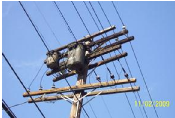
Figure 28: LADWP Pole Mounted Distribution Transformer
