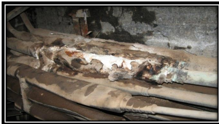
Figure 26: Example of Failed Underground Splice
