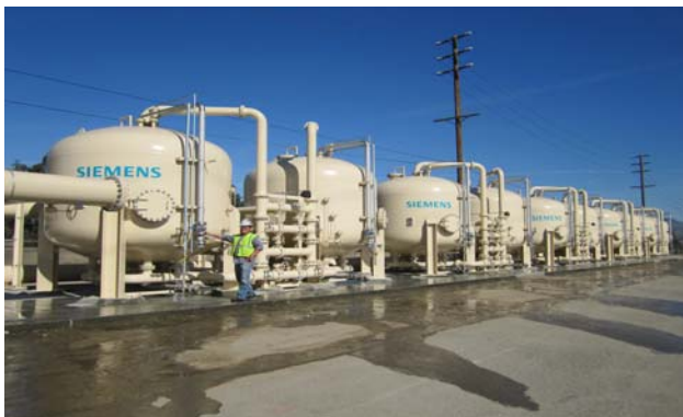
Figure 2: GAC Vessels at Tujunga Wellfield
