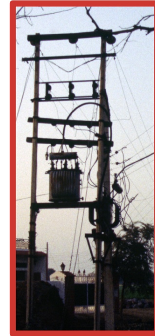
Future Distribution transformer loaded at 145%
