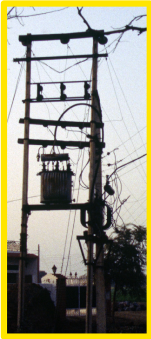
Today Distribution transformer loaded at 115%
