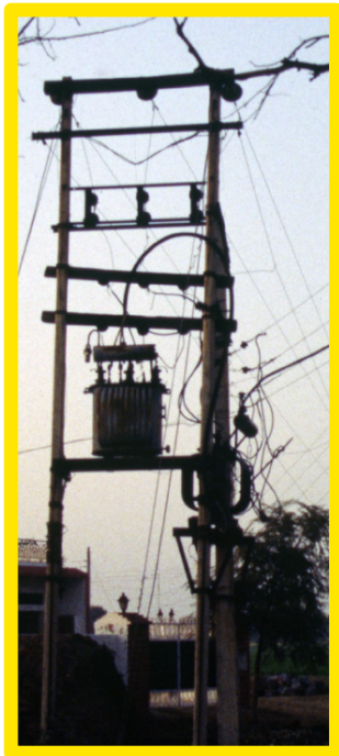
Today Distribution transformer loaded at 115%
