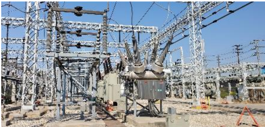
230 kV Circuit Breaker at RS-F
