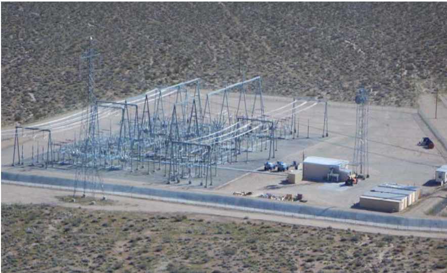
BARREN RIDGE SWITCHING STATION
